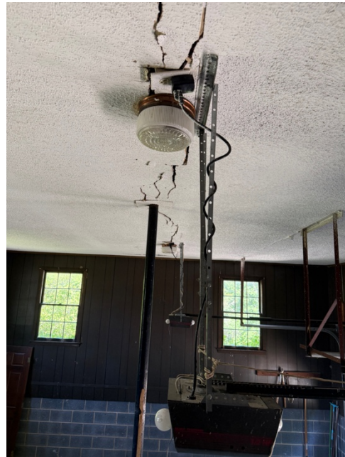
Resulting crack in ceiling
