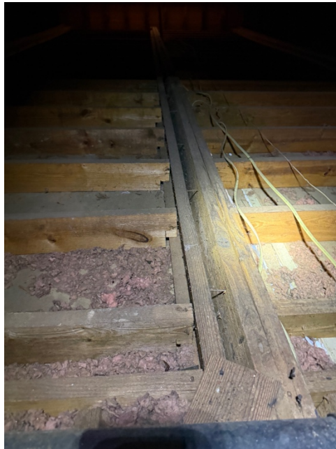
Girder ply separation
